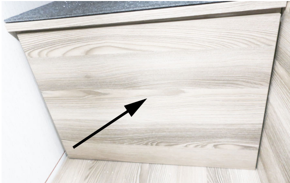
Winterization Valve #1 Pull off the cover to access- located in driver's side rear closet. -Typical View
