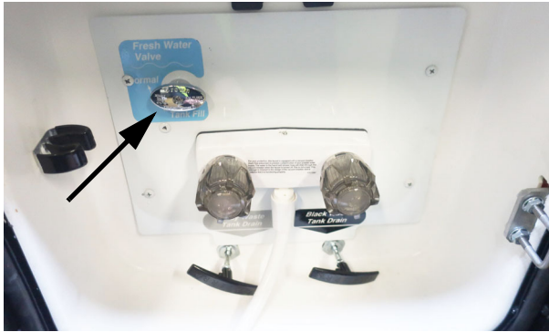
Fresh Water Valve (Located on Water Center Panel shown in normal position). -Typical View
