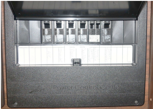
120-Volt Circuit Breakers -Typical View
